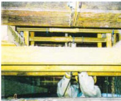
Cutting of tendons between girders after cure of concrete in anchor blocks.
